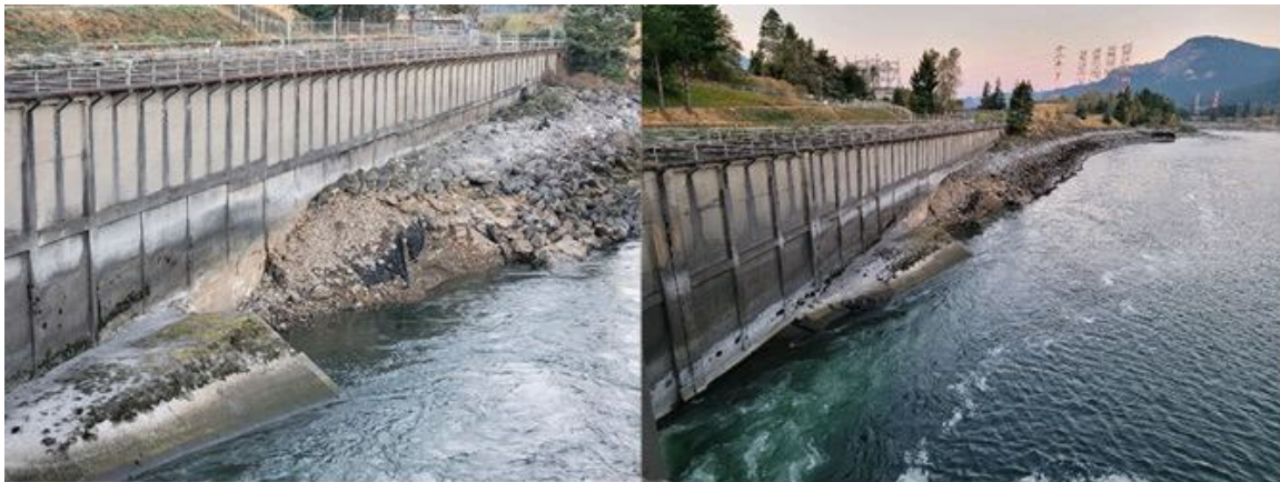
Photo 1: Left frame, close photo of damage to the B-Branch Fish Ladder apron. Right frame, overall photo of the damage. Photo obtained from MOC 22BON089.
